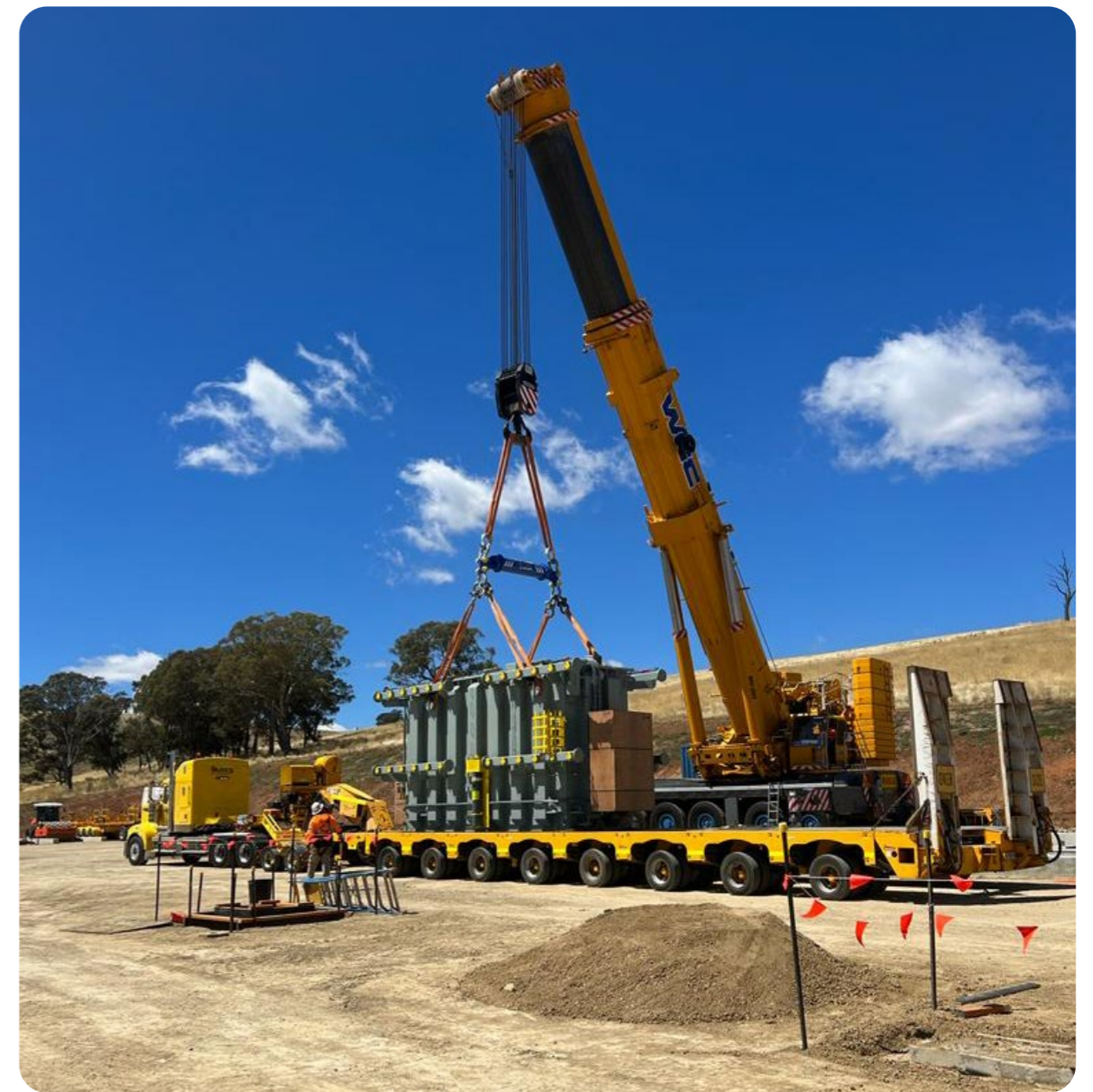
Left: Proposed transport equipment. Above: ARES transporting a 120-ton transformer on a platform trailer.
