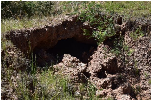
Figure 55: View of clay exposure and extensive sub surface impact within proximity to the transmission tower and in proximity to survey unit 4.
