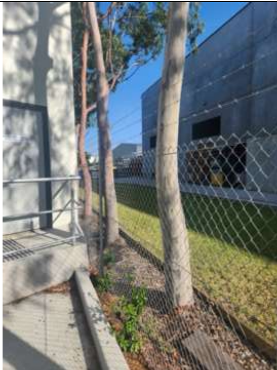
Figure 4 - Photo showing the completed works at 5 Kiora Cres, Yennora, NSW 2161. Image was taken on the 8 March 2024.
