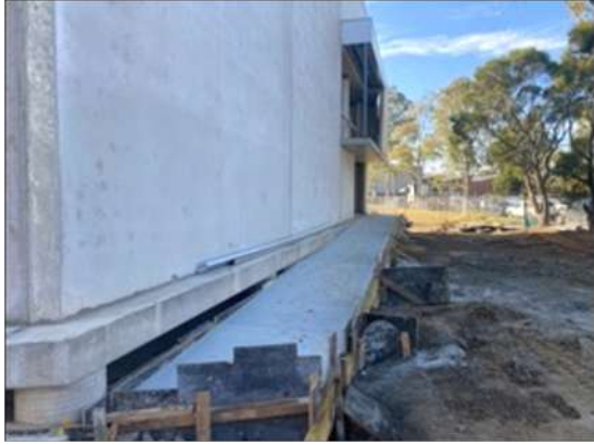
Figure 14 - Photo showing the works located at 5 Kiora Cres, Yennora, NSW 2161. Image was taken on the 8 March 2024.
