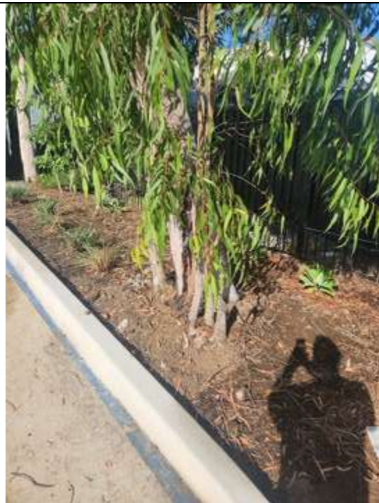
Figure 9 - Photo showing curb & gutter completed works at 5 Kiara Cres, Yennora, NSW 2161. Image was taken on the 8 March 2024.
