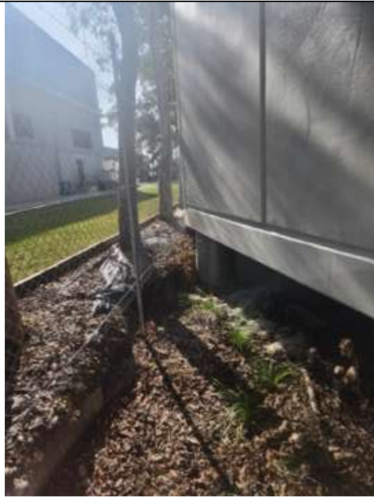
Figure 7 - Photo showing completed works at 5 Kiara Cres, Yennora, NSW 2161. Image was taken on the 8 March 2024.
