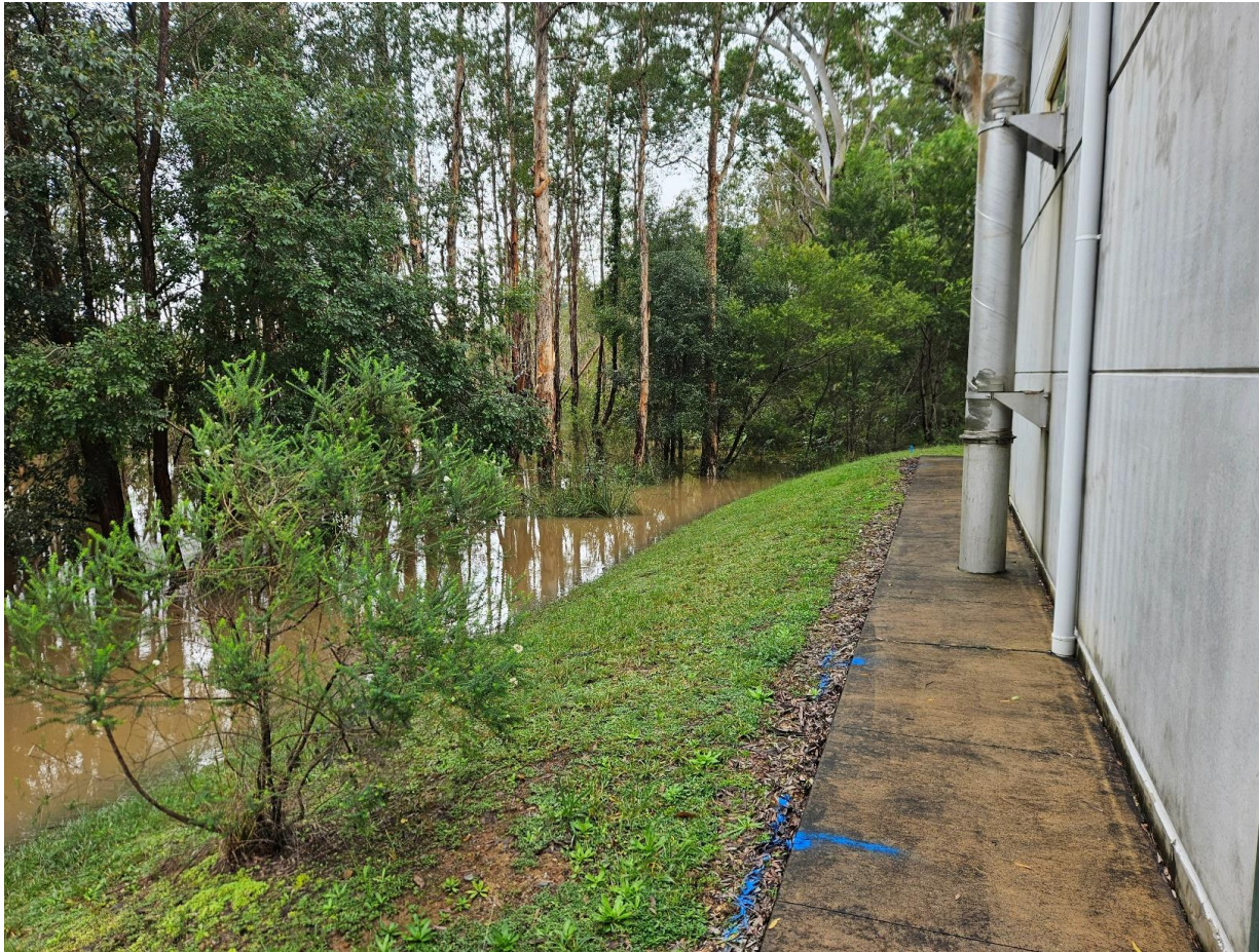
Image 5 Council staff inspection of the Thrumster Sewage Pumping Station #1, 11:04 am 23rd May 2025. Photo looking east-north-east along the northern side of the pumping station building, showing flood waters within several metres of the building. The river levels at the Settlement Point gauge are 0.45 m below the peak level at this stage.
