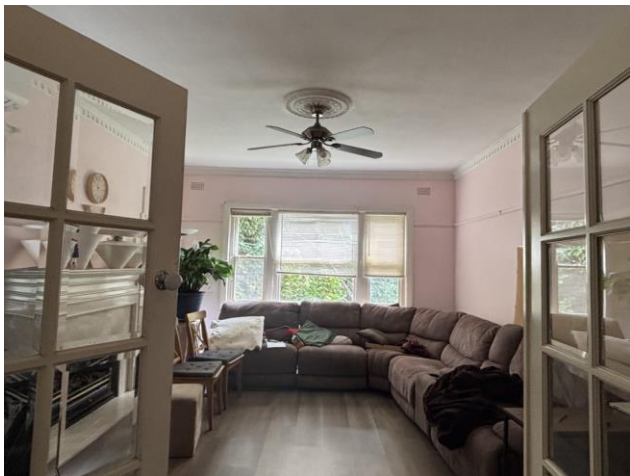
Figure 41 Original sitting room with intact ceiling rose, window, picture rails, air vents and dentilled cornices
