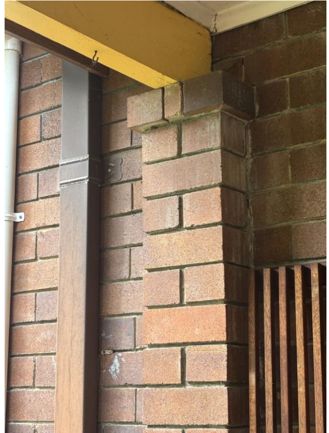
Figure 46 Inconsistency in brick pointing in front area of dwelling indicates potential changes to the brick façade of original dwelling footprint
