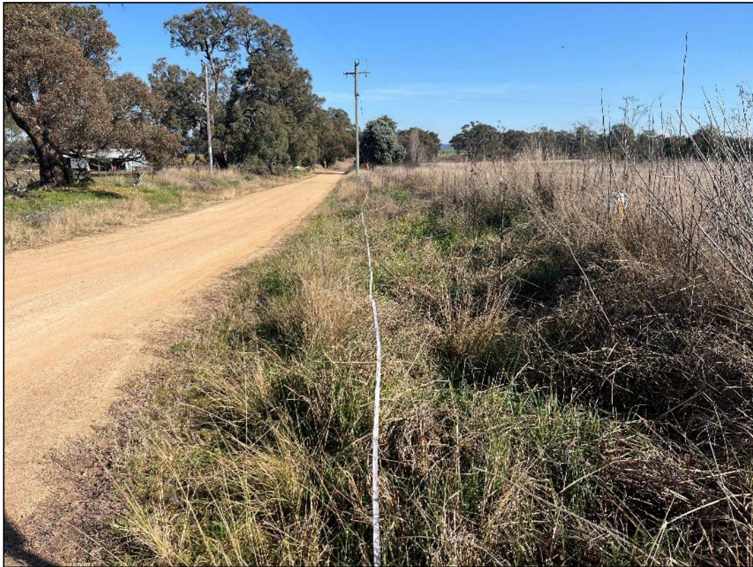
Plate 3: PCT 201 Severely Degraded
