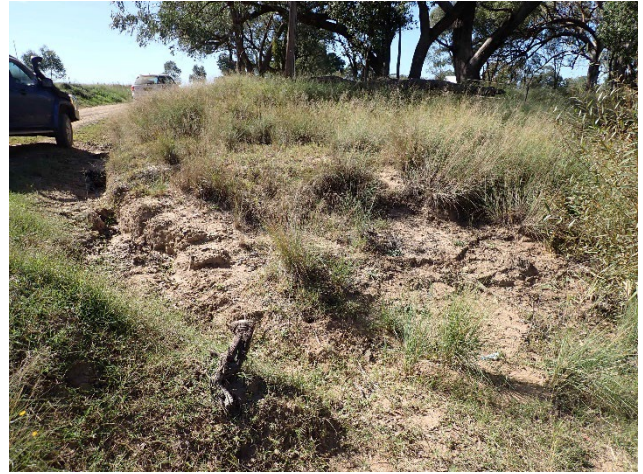
Figure 22 – Exposures adjacent to the creek crossing on Jacksons Lane
