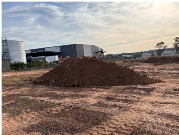
Photo 7: SP25 segregated soil including bulk waste material (3 December 2024)
