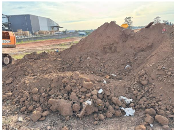
Photo 8: SP25 segregated soil including bulk waste material (3 December 2024)
