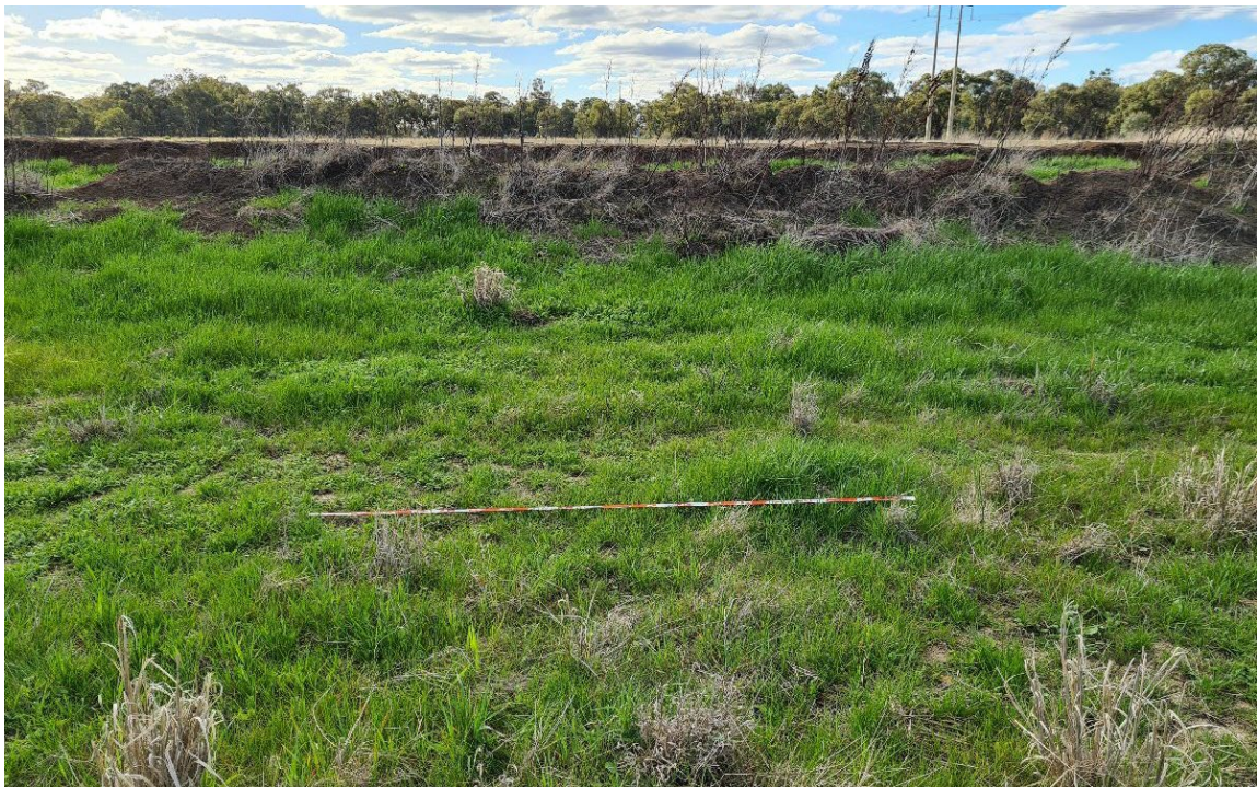
Figure 7.3 North view of channel and levy disturbance near Hartwood Weir. Photograph taken on 13 July 2023 by Nicole Monk.
