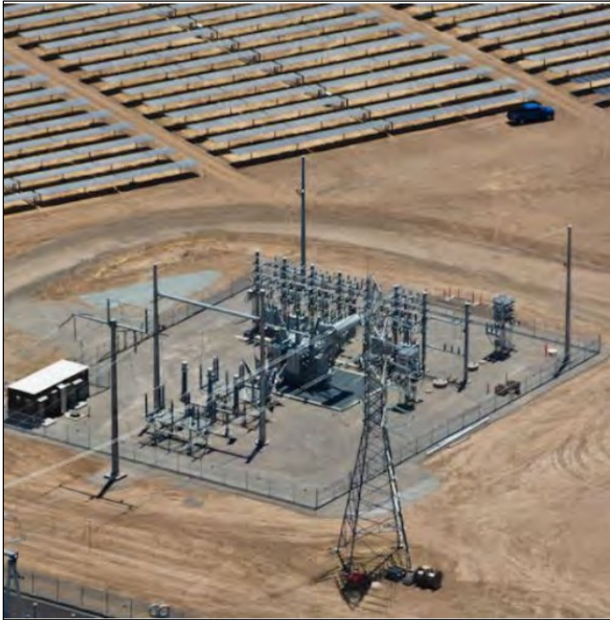
Plate 1: Example Solar Farm Substation Infrastructure and Footprint
