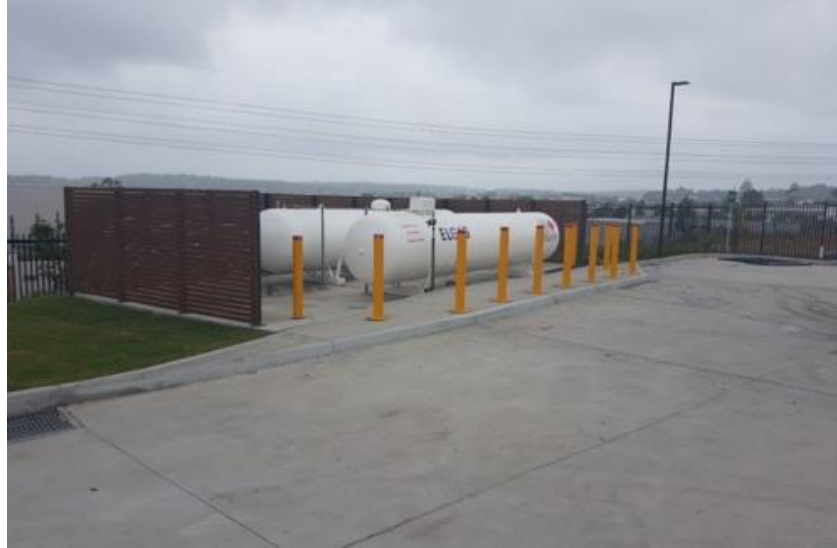
LPG on-site storage tank (reference photo only) – 2 x 7.5kL
