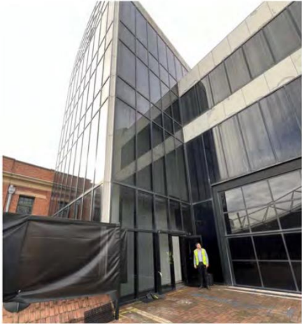
Figure 17: Peeling of the rear façade of the Wran Building
