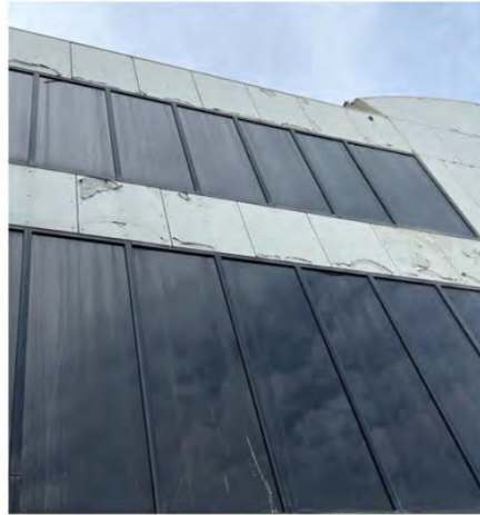
Figure 18: Close up of the peeling façade of the Northern Façade of the Wran Building, including the retrofitted tinting to the glazing.
