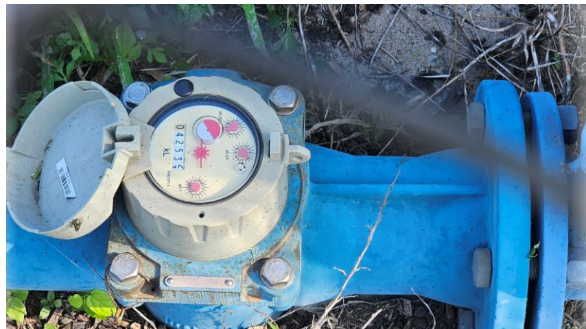
Figure 5 - Existing Water Meter
