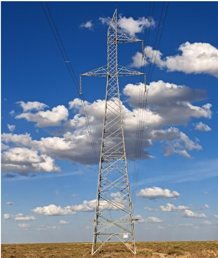
FIGURE 2-5 TYPICAL STEEL LATTICE TOWER STRUCTURE
