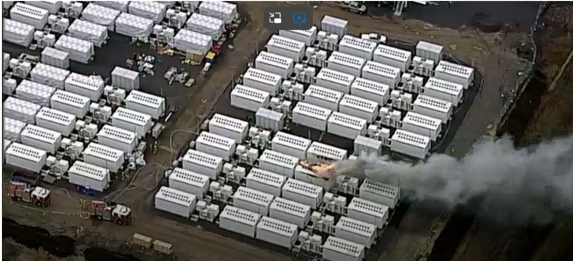
Figure 6: BESS Fire Incident in Victoria, 2021
