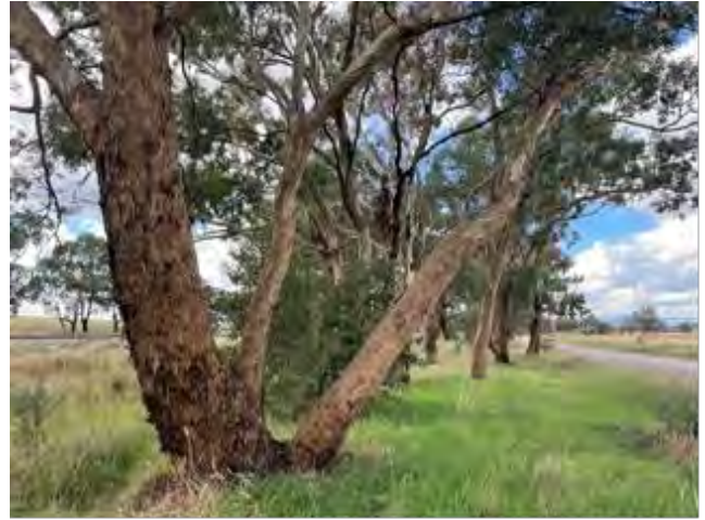
Photo 4.5 PCT 277 poor condition (Q13) along the Junee to Illabo dual track clearances
