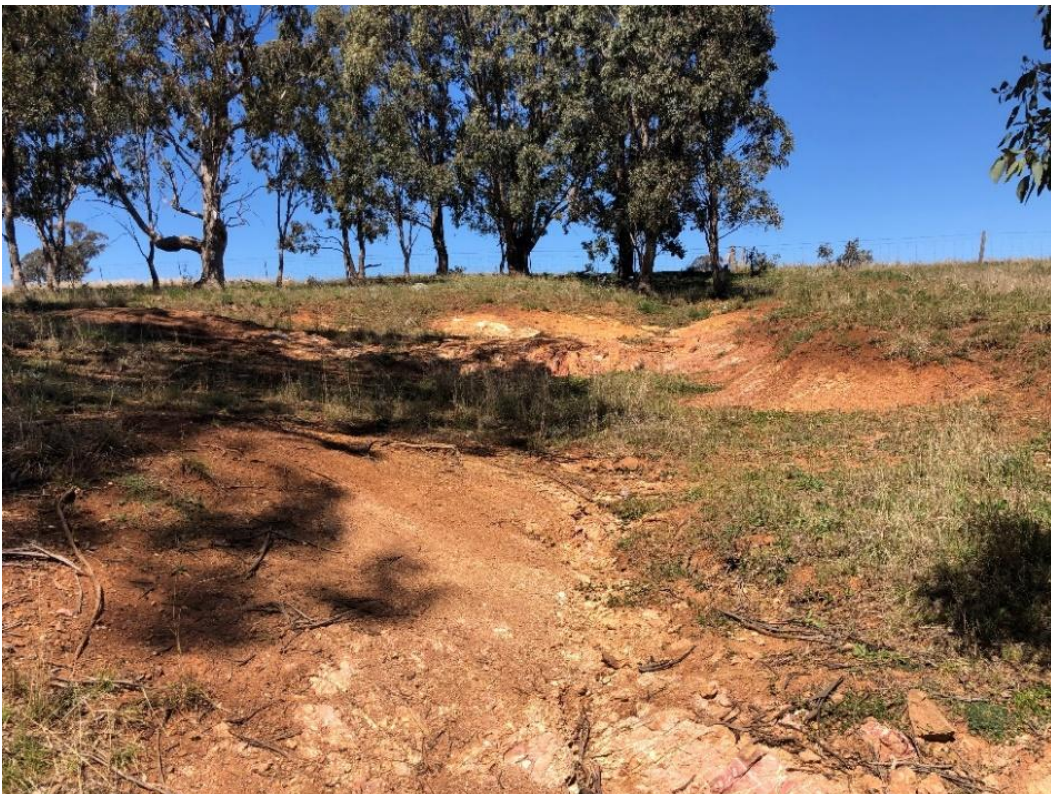
Photograph 4.1 SSF-OS10 showing erosion from water run-off and the depth of soil
