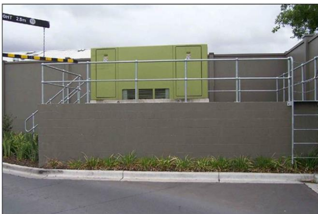
Figure 51 - Example substation raised above 1:100 flood level
