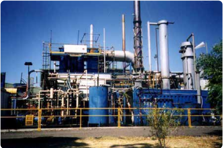
Figure 34: Eli Ecologic Gas Phase Chemical Reduction plant, Kwinana Western Australia. Source: Halett (2013).
