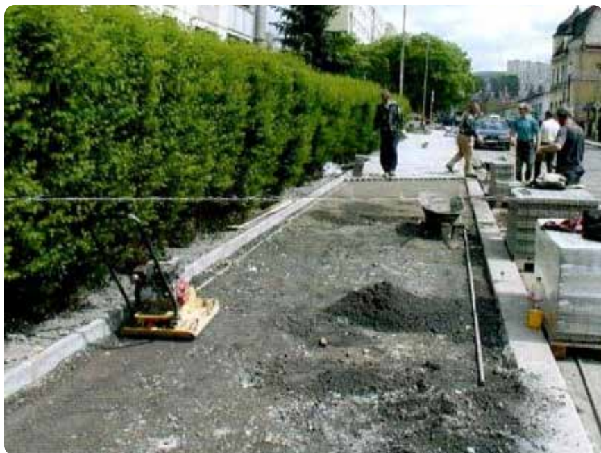
Figure 26: Promotion of use of mixed fly ash and bottom ash as a foundation for sidewalks in the Czech Republic. Levels of PCDD/Fs in this mixture are about 0.05 – 0.1 ppb in WHO-TEQ. Source: Letter sent by company Termizo, operating MWI in Liberec to mayors in the region.
