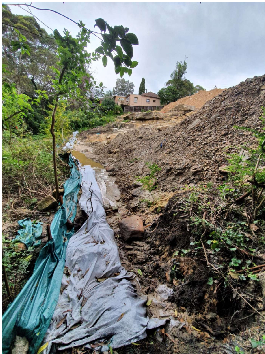
Photo1: Steep slope of unconsolidated excavated rock and sediment with a totally inadequate low silt fence on the edge of bushland reserve
