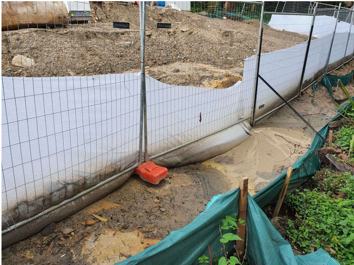
Photo 2: A single layer fabric-lined steel fence can also be breached in extreme weather. A second layer is required to act as a failsafe. For either fence on a steep slope the traditional low green fencing is totally inadequate.
