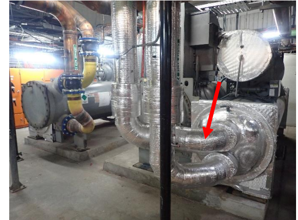
Photo 27: Harbourside – assumed SMF insulation to Chillers #3, #4 and #5 in the chiller plant room on Level 1
