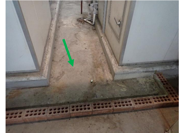
Photo 39: Harbourside – non-asbestos containing cream fibrous membrane between AHU 3.1 & 3.2 in the plant room on Level 3
