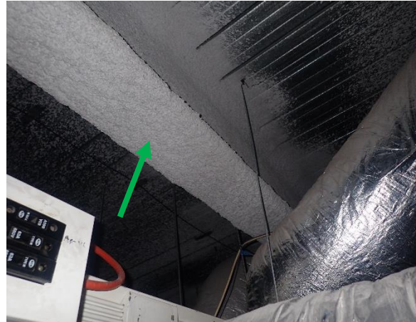
Photo 32: Harbourside – non-asbestos containing vermiculite to the steel beams within the ceiling cavity of Shop 316 (formerly Racecentre) on Level 2
