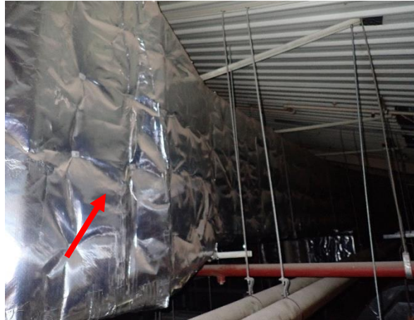
Photo 50: Harbourside – assumed SMF insulation to the HVAC ducting in the plant room on Level 3
