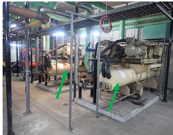
Photo 23: Harbourside – non-lead based cream paint to Chillers #1, #2 & #5 in the chiller plant room on Level 1
