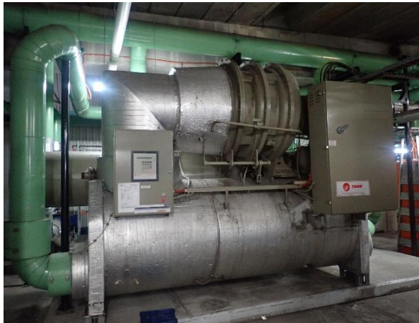
Photo 16: Harbourside – assumed asbestos containing gaskets to Chiller #5 in the chiller plant room on Level 1
