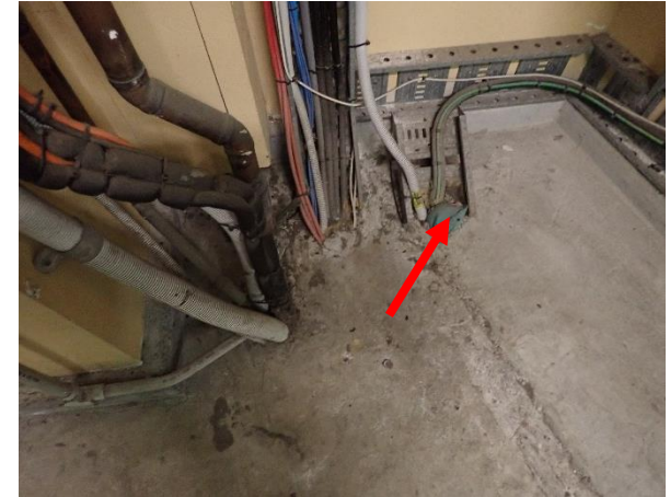
Photo 51: Harbourside – assumed SMF insulation to packing pillows
