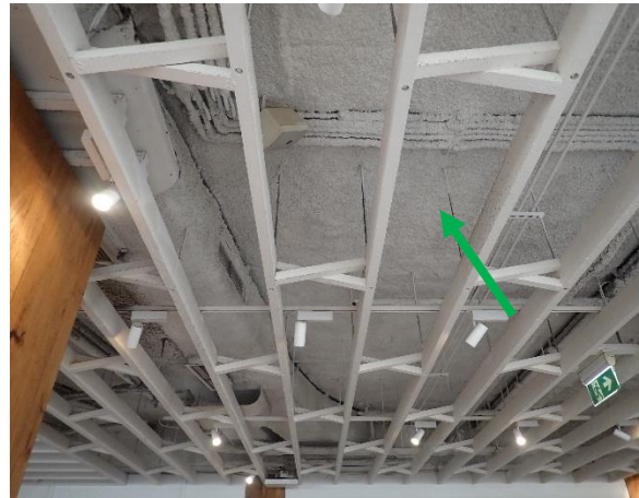
Photo 17: Harbourside – non-asbestos containing vermiculite to the steel beams & ceiling in Shop 198 (Cyren) on Level 1
