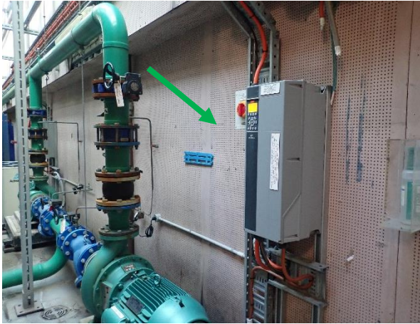
Photo 43: Harbourside – non-asbestos containing fibre cement sheeting to the walls of the cooling tower area on Level 3
