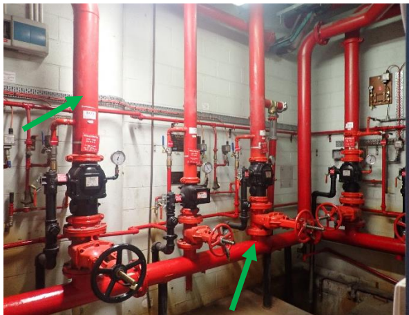
Photo 22: Harbourside – non-lead based red paint to the pipework within the sprinkler valve/pump room on Level 1
