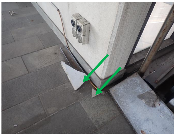
Photo 58: Former Monorail Station – non-asbestos containing compressed fibre cement debris to the station platform
