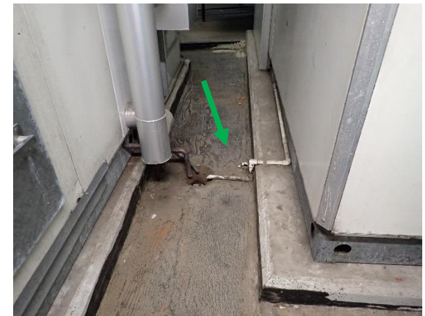
Photo 42: Harbourside – non-asbestos containing black membrane between AHU 3.3 & 3.4 in the plant room on Level 3
