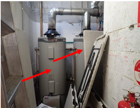
Photo 28: Harbourside – assumed SMF insulation to the hot water systems within the tenancies on Level 1
