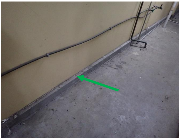
Photo 40: Harbourside – non-asbestos containing white caulking to the base of the south wall in the plant room on Level 3
