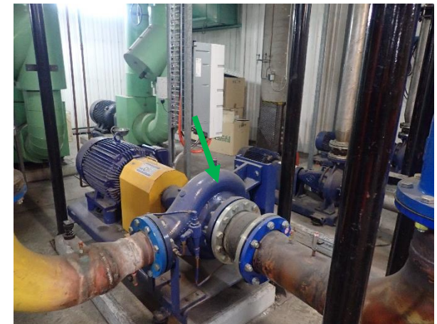
Photo 24: Harbourside – non-lead based blue paint to the pumps in the chiller plant room on Level 1
