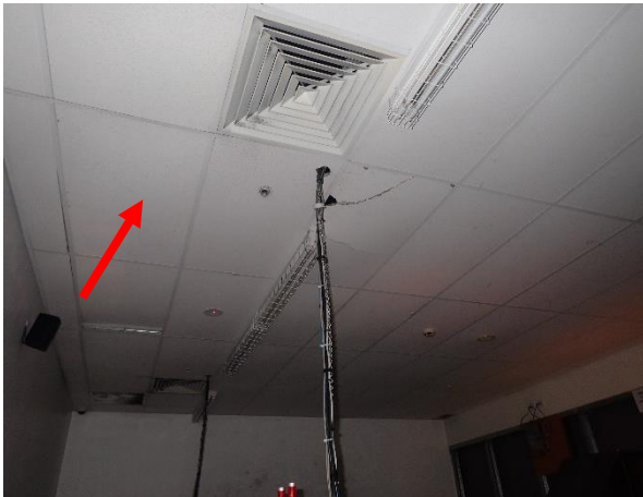
Photo 52: Harbourside – assumed SMF suspended ceiling tiles to the bowling machine rooms in Shop 501 & 502 (Kingpin) on Level 3
