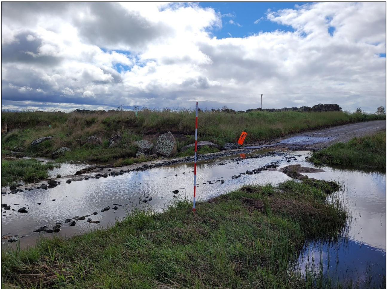
Figure 1-14 Damaged low-level crossing over Blind Creek. This crossing would require repair
