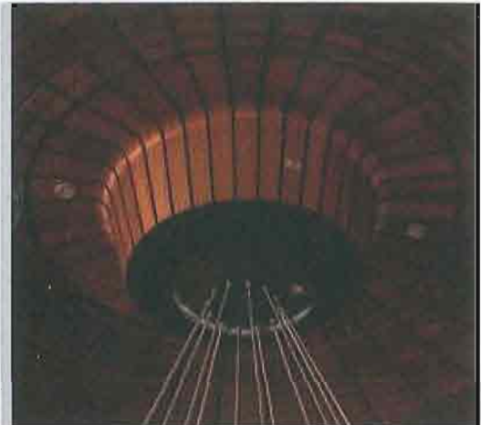
Figure 23 Detail of the timber element holding the central chandelier in the Wool room (FS 2011).
