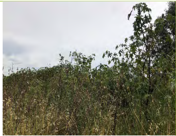
Photo 12. Weed growth on crest of bund
