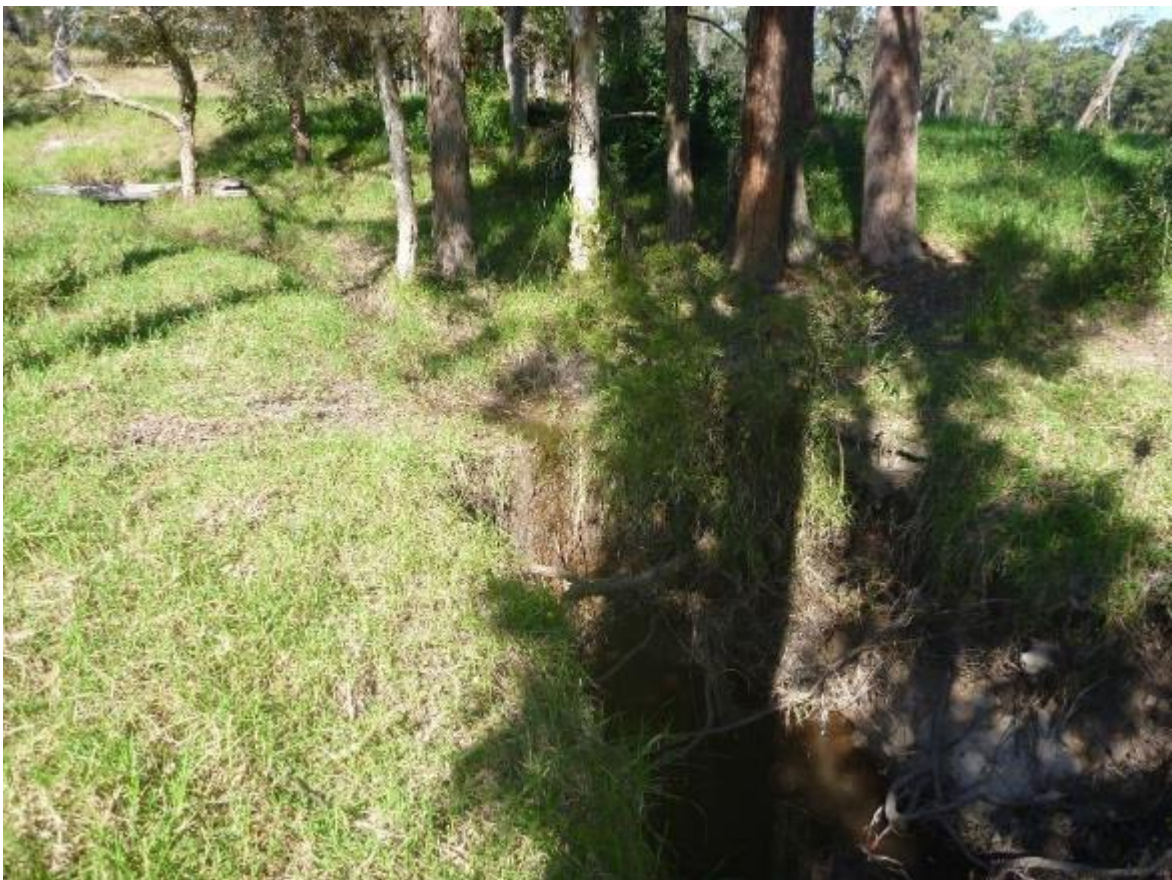
Plate 32: Looking upstream at the upstream limits of the deeply incised, sunken channel headcut.
