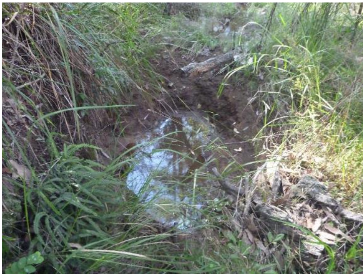
Plate 20: Typical scour pool in the channel area downstream of Deep Creek Rd crossing in ST4.
