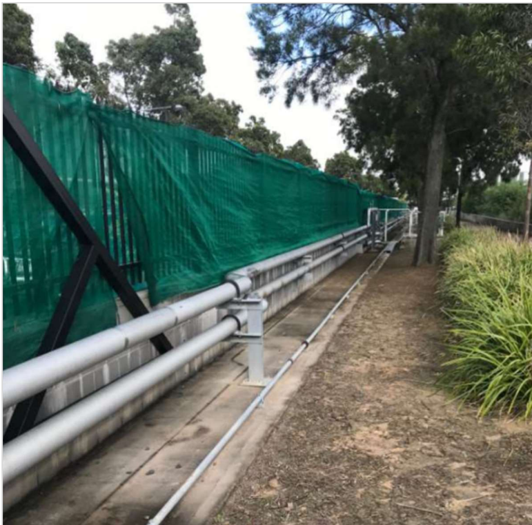
Figure 1: Infrastructure associated with the Botany Groundwater Clean-Up Project (Source: Keylan)
