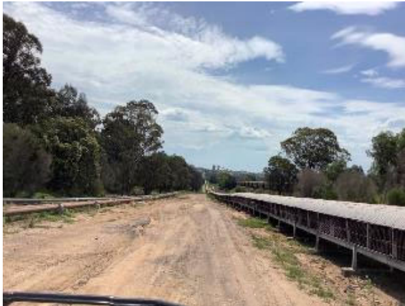
Photo 5-12: Cleared corridor containing the eastern coal conveyor and access track. Native trees are situated beyond the edge of the development site.
