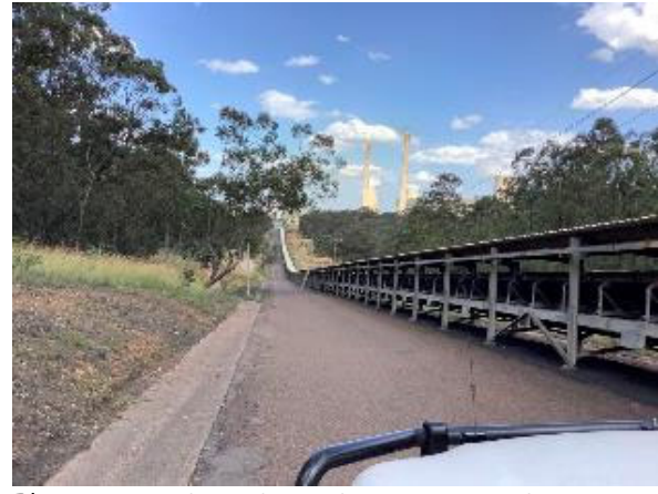
Photo 5-13: Cleared corridor containing the western coal conveyor and access track. Native trees are situated beyond the edge of the development site.
