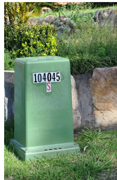
Underground service pillar
