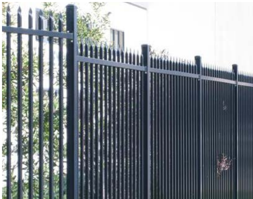
1.8m Security Perimeter Fence
