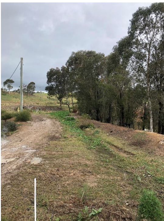
Figure 4 Stormwater diversion drain along the eastern side of leachate dam (south west direction)
