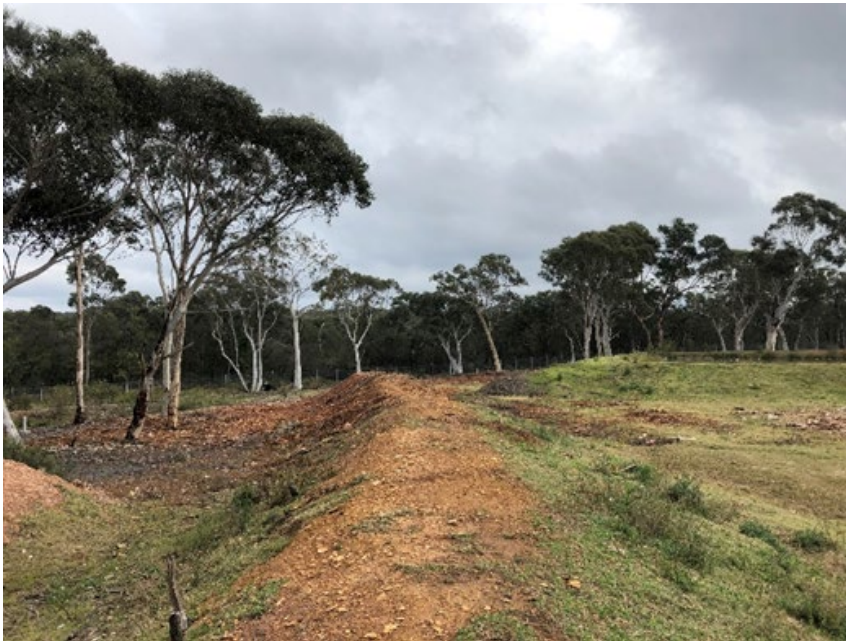
Figure 11 Stormwater discharge area - diversion of stormwater near the stormwater dam – north west direction
