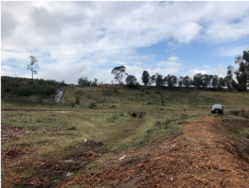
Figure 9 Stormwater System collecting run-off from the higher ground of Stage 1 and diverting past the leachate dam embankment – east direction
