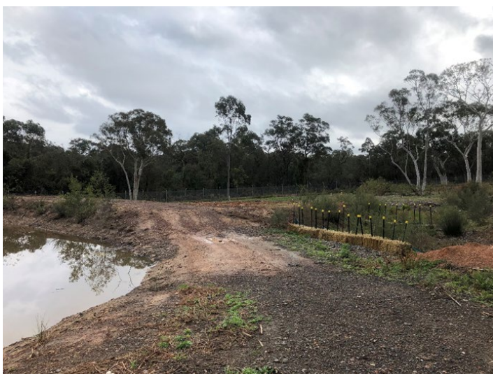
Figure 6 Leachate Dam (low end point) with the discharge point and associated operational structures to stop overflow (west direction)
