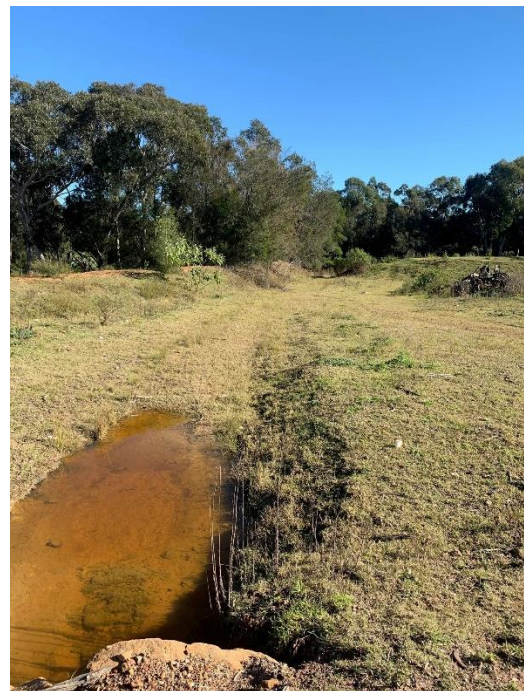
Plate 20 – Stormwater Drain Outlet (Below Drop Down Drain)
