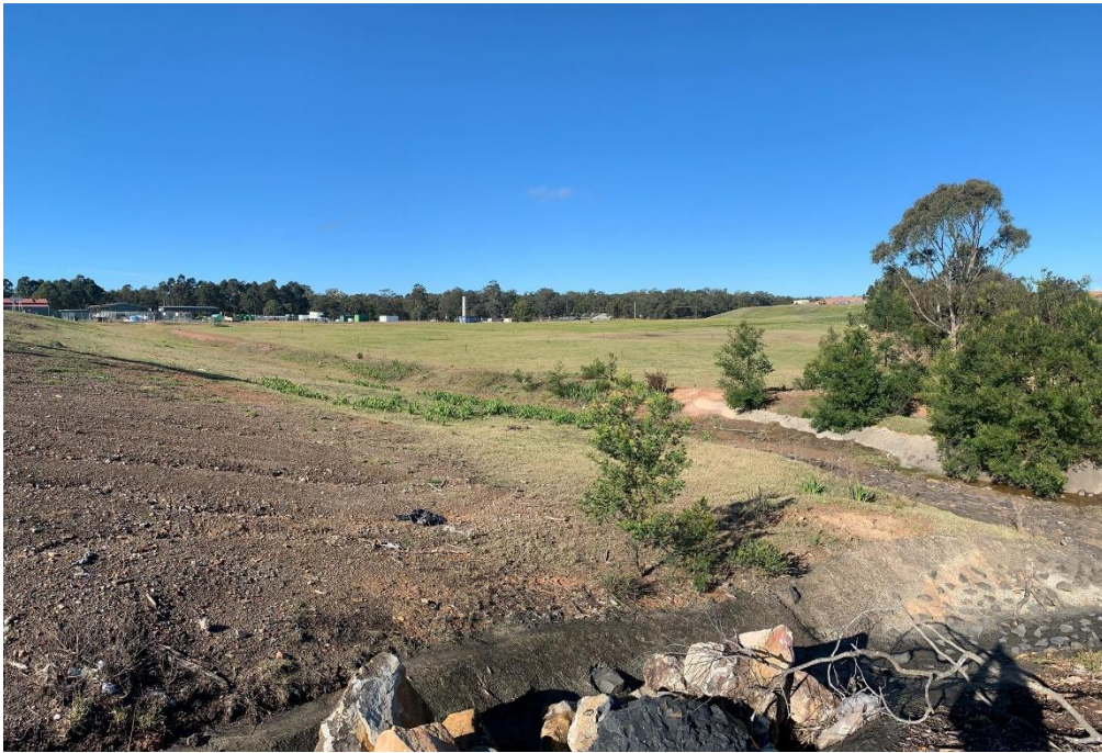
Plate 21 – Irrigation (Utilisation) Area with Stormwater Drain in Foreground
