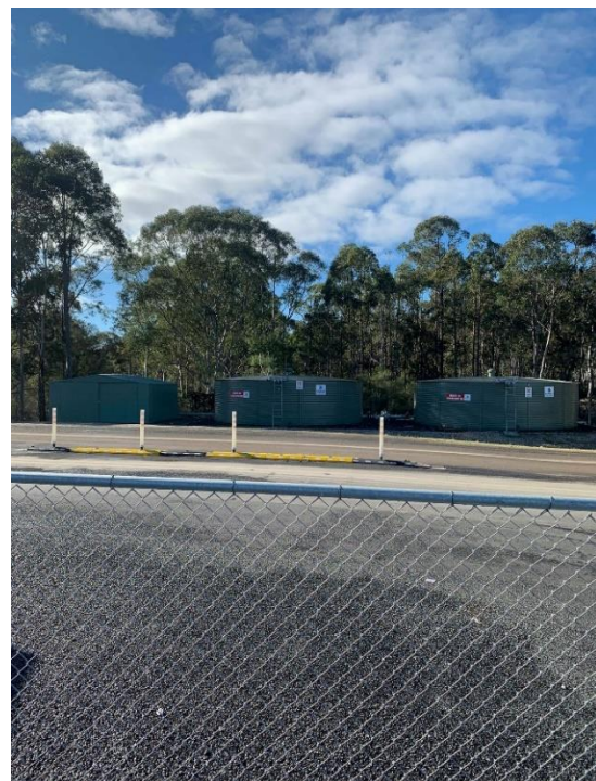
Plate 4 – Water Tanks [Fire-Fighting Capacity]
