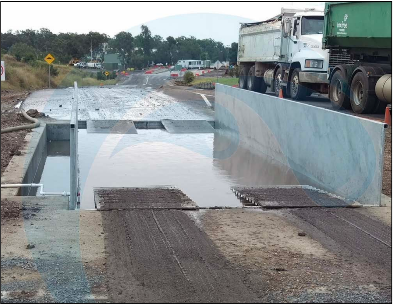
PHOTOGRAPH 4.2: Typical wheel wash, to be employed the site.
