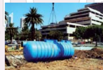
SPEL STORMCEPTOR™ treating stormwater from various carparks and streets in PERTH CBD - Perth City Council.
