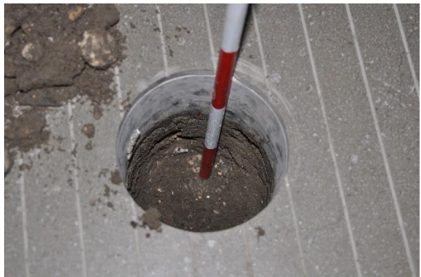
Figure 4.6 Example of one of the boreholes excavated onto sandstone bedrock. (Source: GML, 2019)
