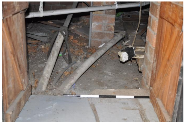
Figure 4.4 View under the current building showing concrete and building footings. (Source: GML, 2019)
