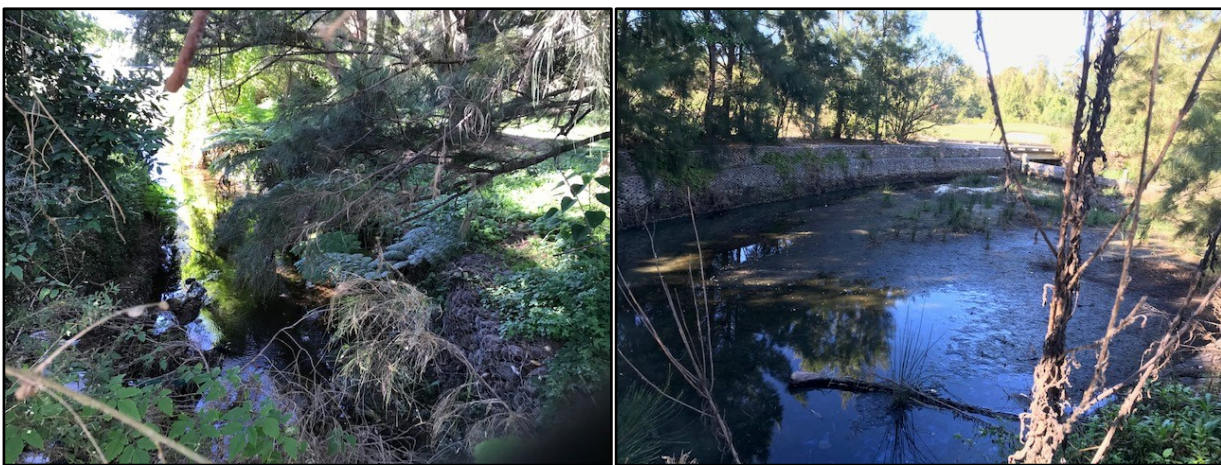
Figure 3-18 Modified sections of Burnt Bridge Creek near Manly Golf Course (Photo date: 26/05/2021).
