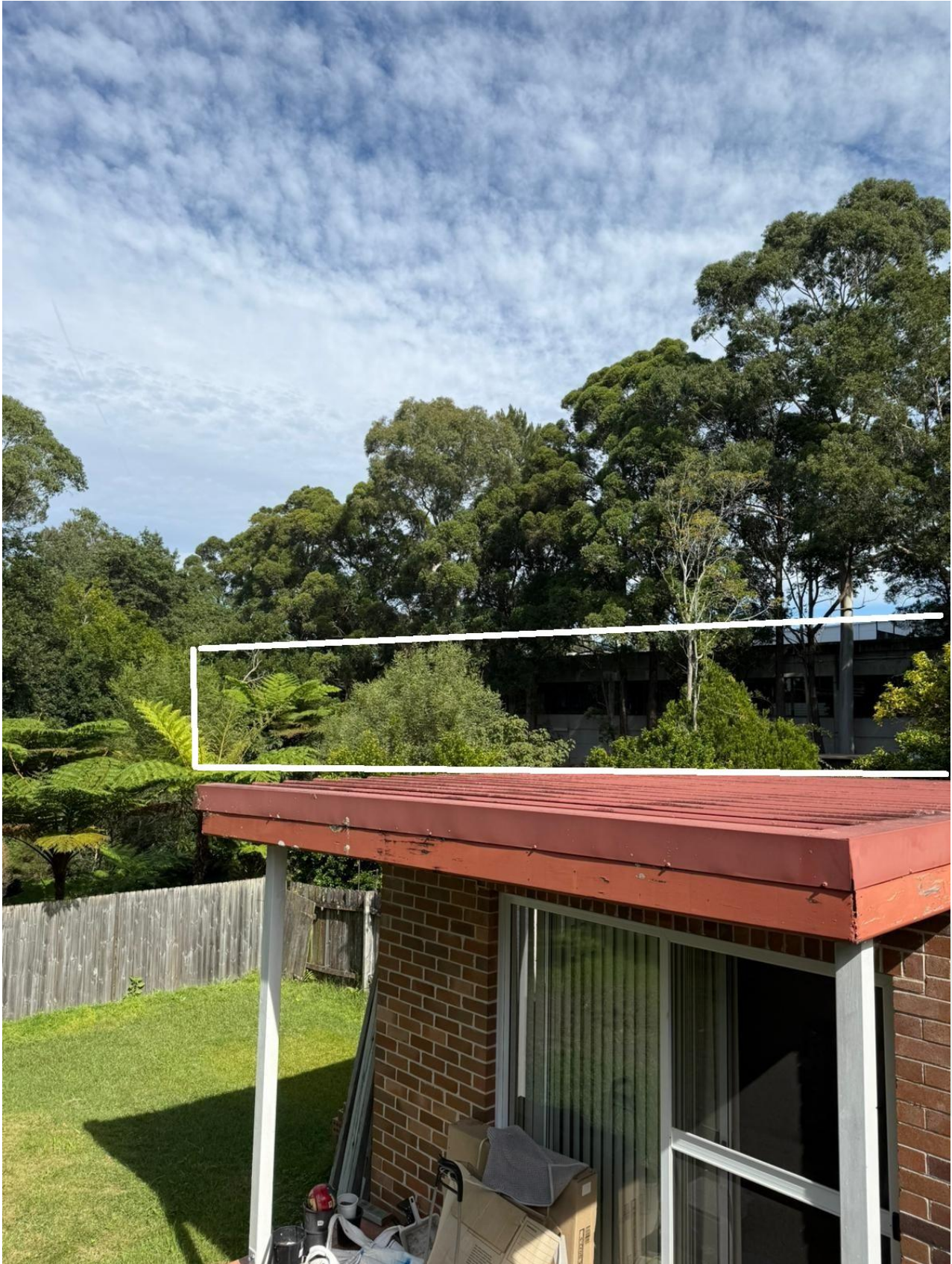
Figure 15: Rear yard of 8 Banksia Close, existing structures shown in white. (Source: Council Planner)
