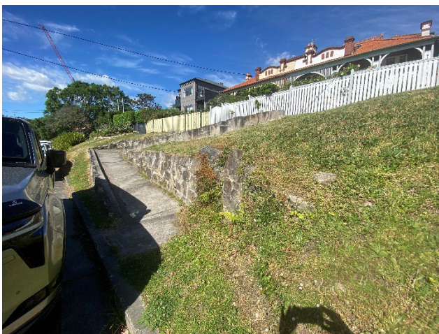
Figure 8 Retaining wall, concrete path cut through it.
