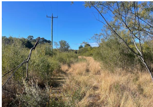
Figure 12: Clearance below power lines
