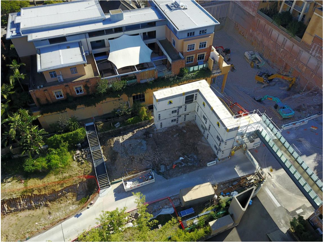
Figure 3 - Aerial view of STEM building construction site with northern end of 52 McLaren Street in foreground (Source: Wenona)
