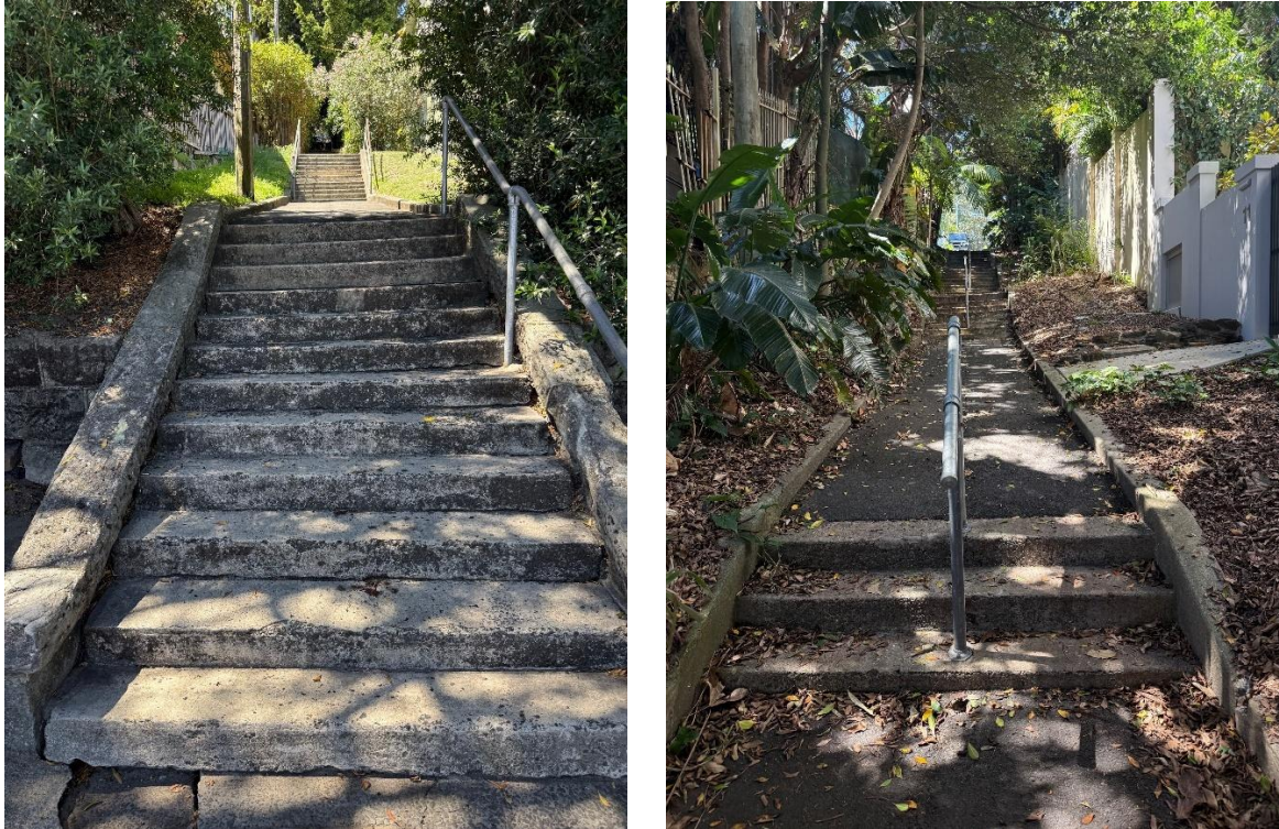
Figure 3: Images of the footpath that connects Fernleigh Avenue to New South Head Road, Rose Bay Source: Council Staff
