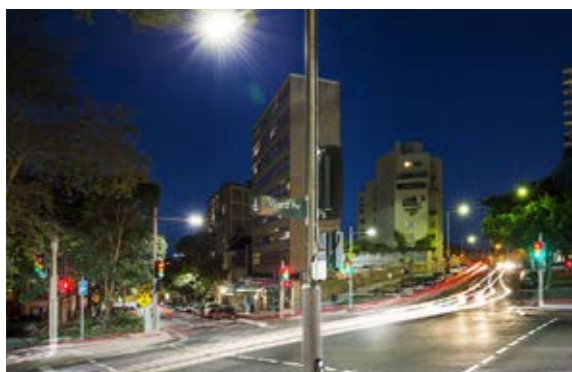
City of Sydney Light Pole
