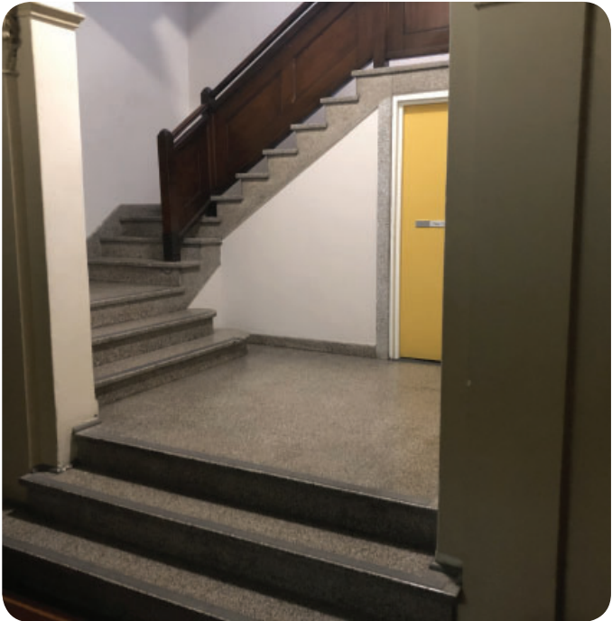
The main entry and foyer from Forbes Street incorporate a number of steps and level changes that do not allow disabled access through the main entry of the building. Access throughout the building does not meet contemporary requirements.
