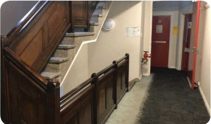
Access within Wilkinson House is via a narrow circulation stair (900mm) that does not cater for the volume of students moving between classes and results in a bottleneck.
