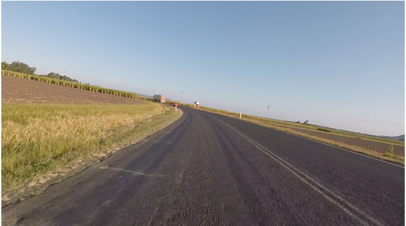
Photo – Skid marks from a heavy vehicle on Woodburn Coraki Road approaching Reardons Lane
