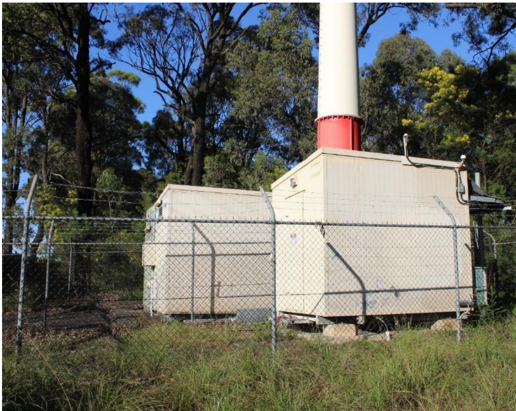
Plate 2. Telecommunications facility adjacent to the eastern fence in SU1, view to south. (Source: Heritage Now 2025)
