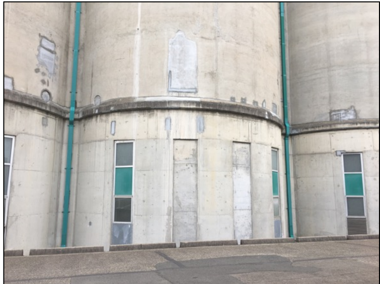
Figure 21: Previous patching work on the northern side of the silos.
