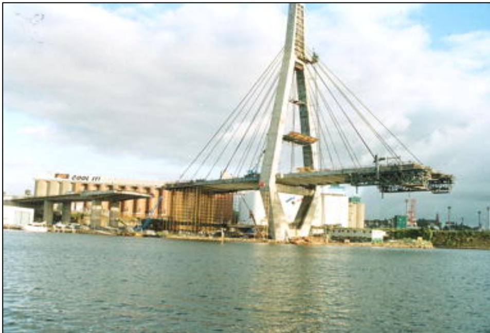
Figure 7: The Anzac Bridge under construction, the c.1975 Silos are in the background.
