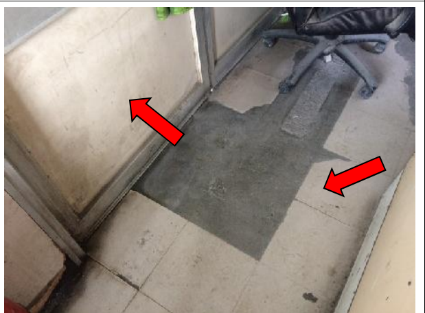
Photo 27: Asbestos containing vinyl floor tiles and asbestos cement sheet infill door panels in the weighbridge offices
