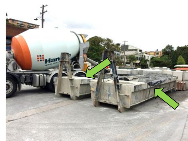
Photo 8: Waste bins for waste concrete from returning trucks
