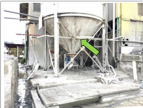
Photo 1: Wash out pit area with solid slurry and liquid waste tank
