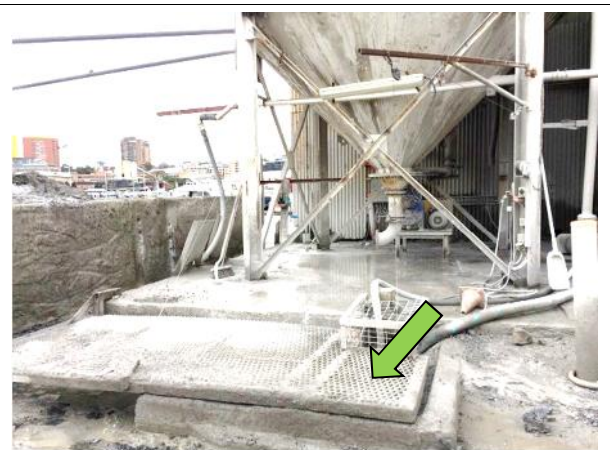
Photo 2: Sump pit for collection of liquid waste from the washout pits
