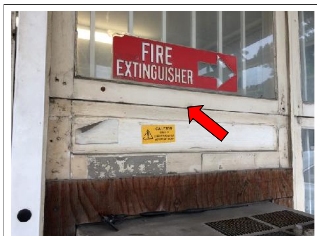
Photo 31: Main Office Building, Exterior Window Frames – 'Leadcheck' tested positive for lead
