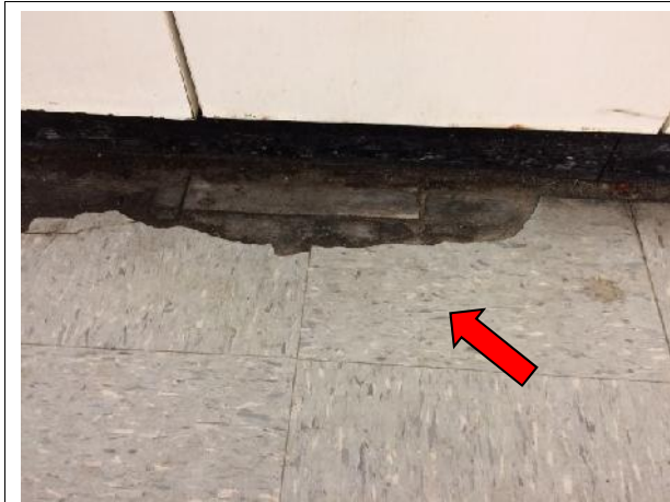
Photo 24: Asbestos containing vinyl floor tiles (lower older layer) in the lunch room of Amenities Building
