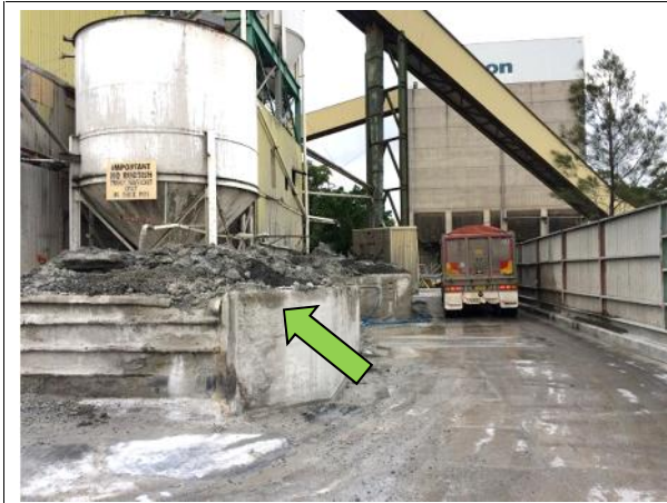
Photo 10: Wash out pit area with solid slurry and liquid waste collection/reuse tank
