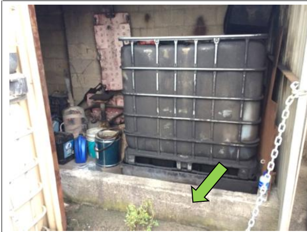
Photo 6: Waste oil from site processes stored in a intermediate bulk container (IBC) within bunding
