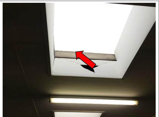
Photo 23: Damaged asbestos containing fibre cement sheet skylight panelling in the lunch room of Amenities Building
