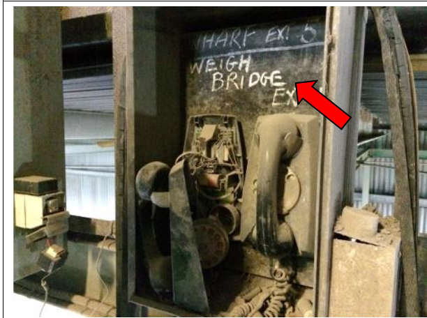
Photo 26: Asbestos containing backing board behind phone in area above the silos
