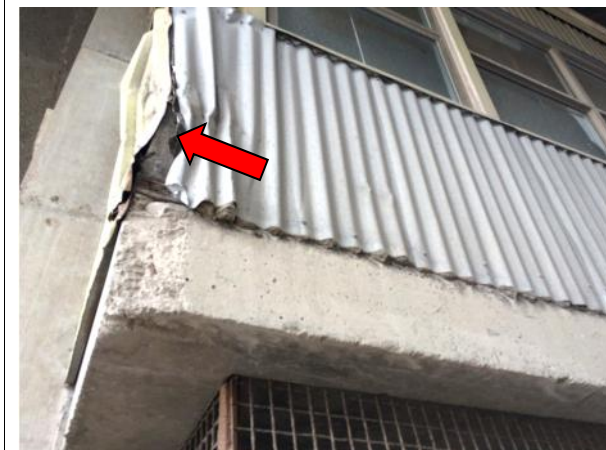
Photo 30: Exterior, Weigh Bridge Offices, Lower Wall Sections behind metal sheeting – Suspected SMF insulation
