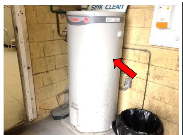
Photo 29: Exterior, adjacent Lunch Room Entrance – Suspected SMF internal insulation
