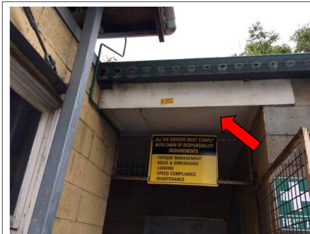
Photo 22: Asbestos containing fibre cement sheet ceiling and wall panelling of entrance awning to Amenities Building
