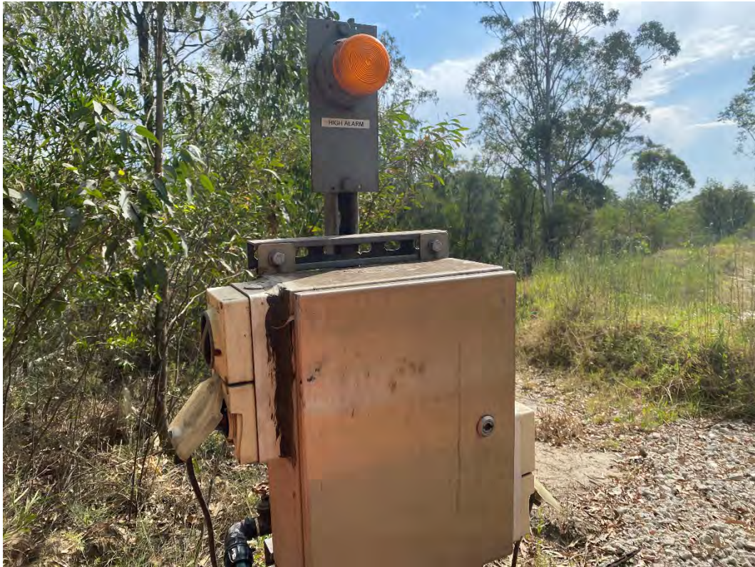
Plate 19 – Trade waste pump with high level alarm
