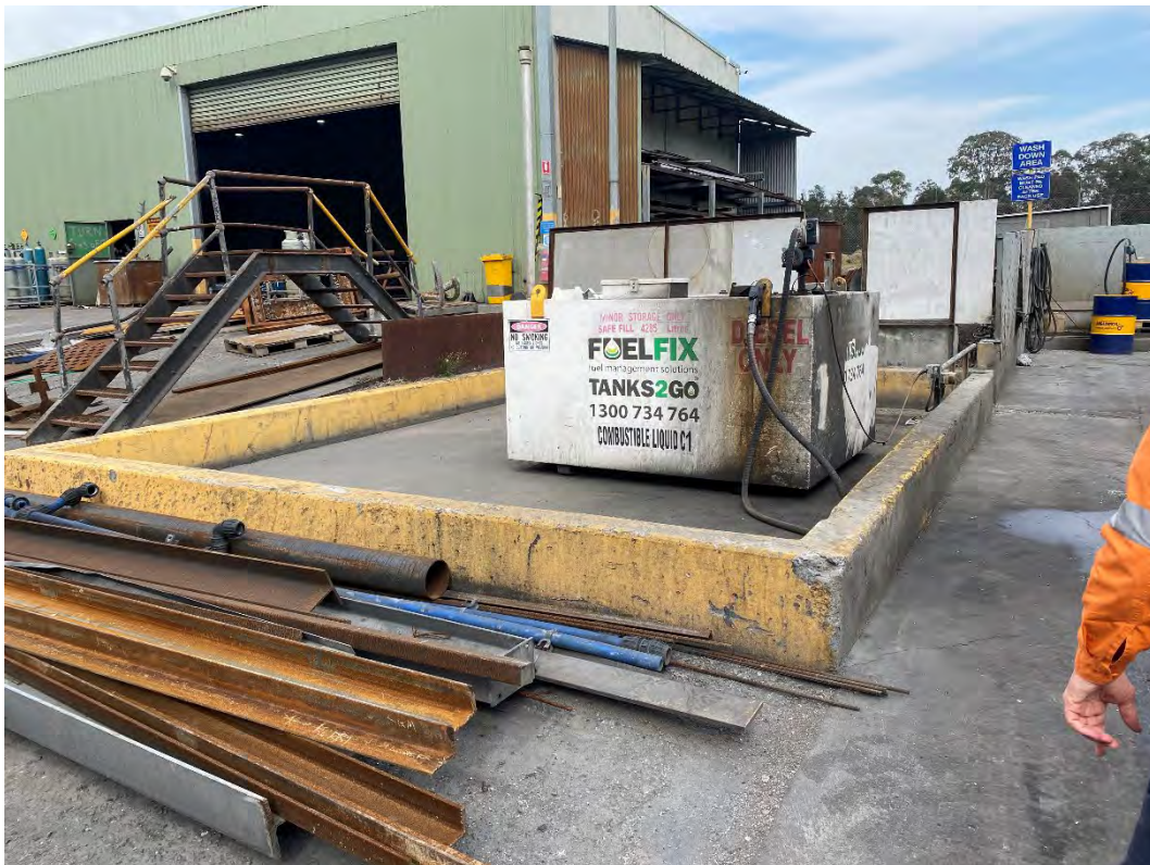
Plate 14 – Double skinned fuel tank with concrete bunding
