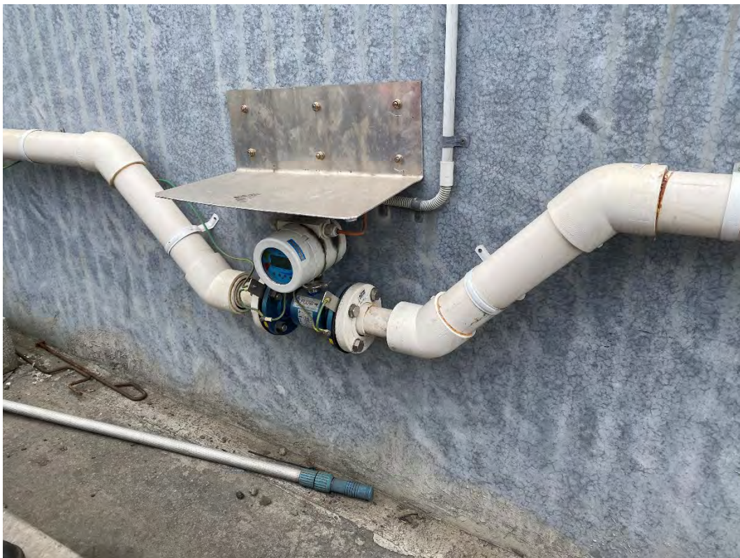
Plate 20 - Mag flow meter (reports to Hunter Water)
