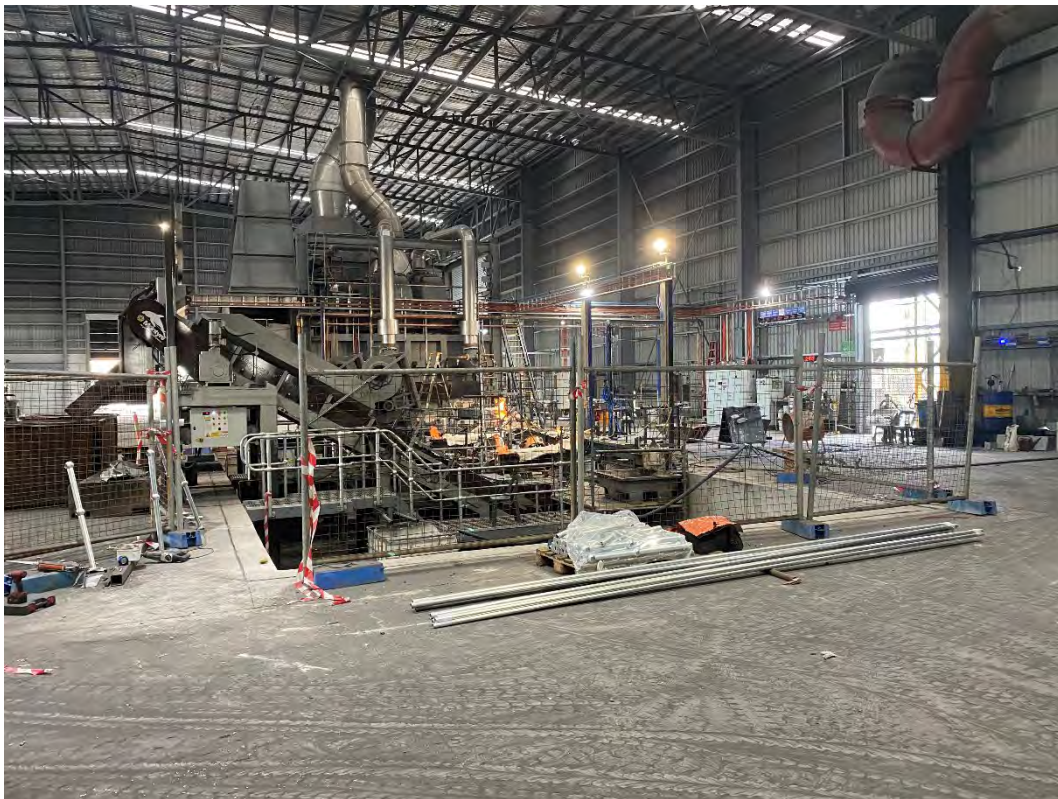
Plate 5 - Casting lines with extractors to Baghouse 1 in background
