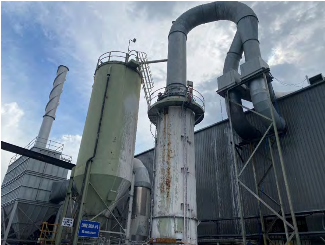
Plate 11 - Lime Silo No. 1 with furnace ventilation in foreground
