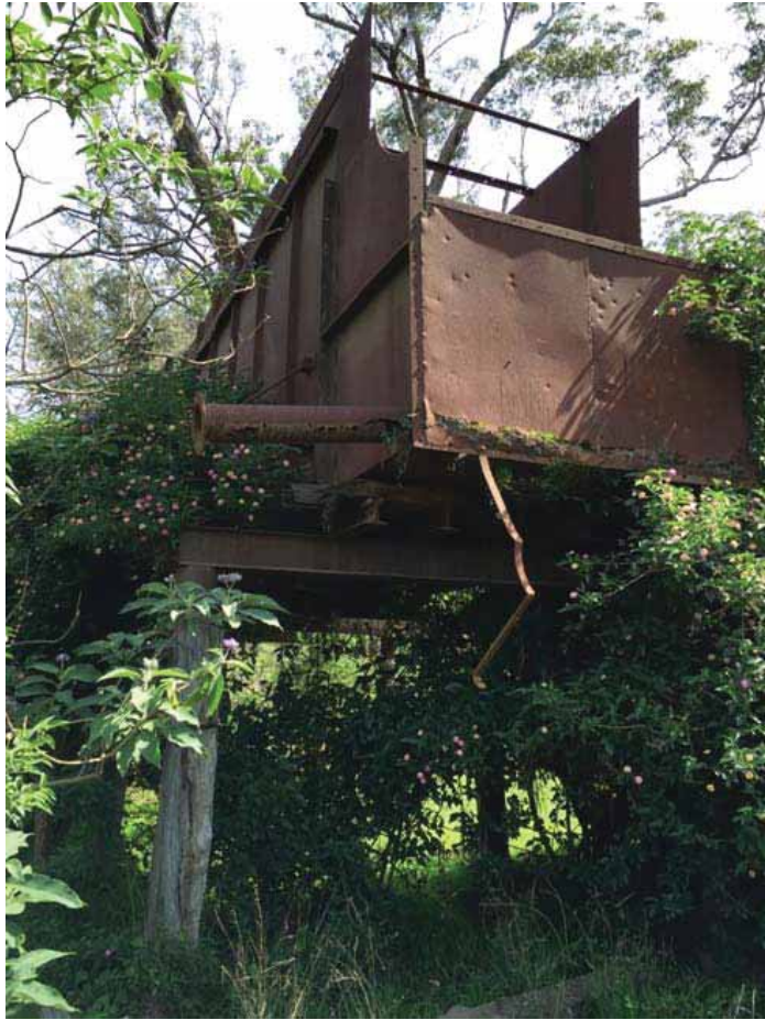
Plate 4.1 Close up of the loading bin showing possible drainage spout from north-east corner, railway sleepers tracks.
