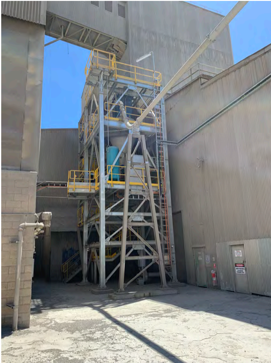
Figure 1.2: View of the satellite section of the Chloride Bypass System near CM5 and CM7
