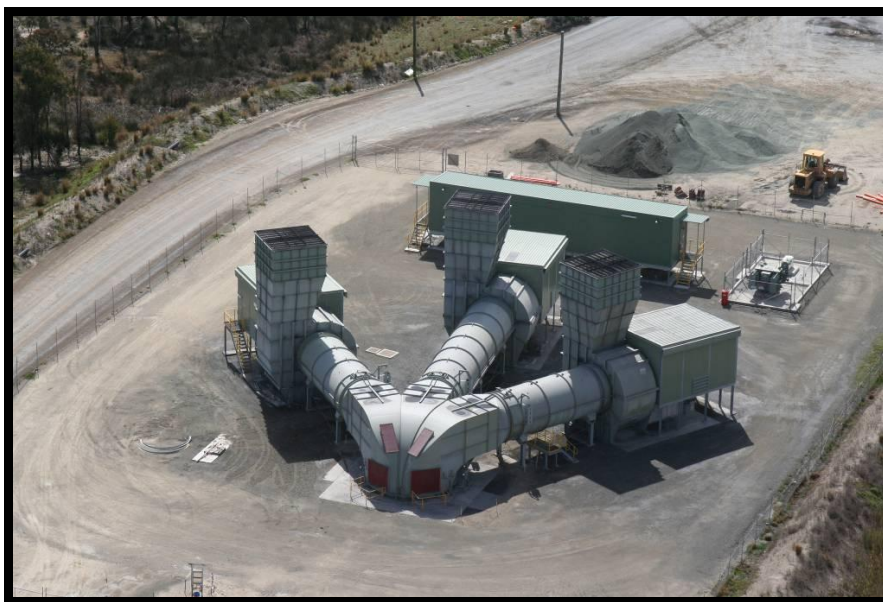
Plate 7 – Existing upcast ventilation fan at Blakefield South Underground Mine.
