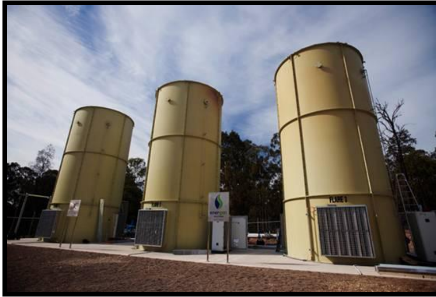
Plate 2 – Existing Gas Flares at the BFS Underground Mine
